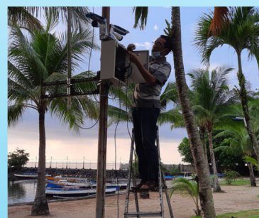
Tasik Ria Resort - CCTV
