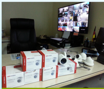
Bank BNI 46 CCTV
