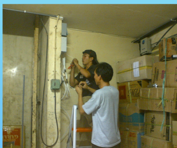
Golden Supermarket- Alarm System
